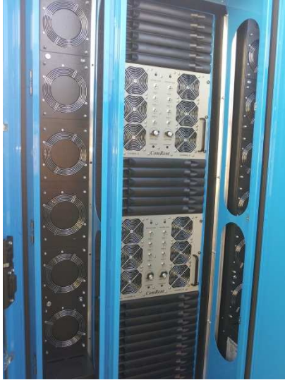
R.A.S.E.R. HD 23Kw of Load Bank
