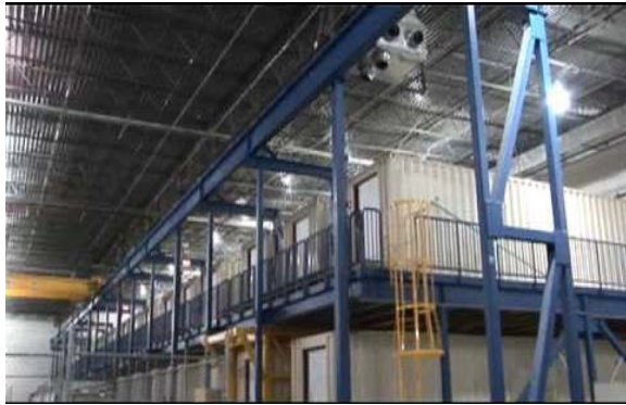
Figure 2: Data Center Featuring Container Units - Oregon
