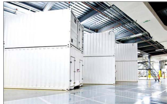
Figure 3: A Chicago Area Data Center Featuring Stacked Container Units
